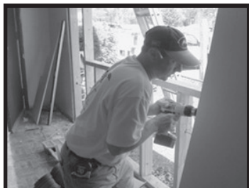
Volunteers not only make home repairs but also get the chance to meet members of their community: homeowners and other volunteers.
