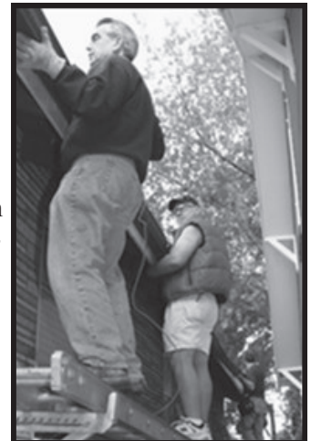
A team of volunteers working on the side of a house. RT works to make homes, like that of Mrs. Moore, safe and secure.
